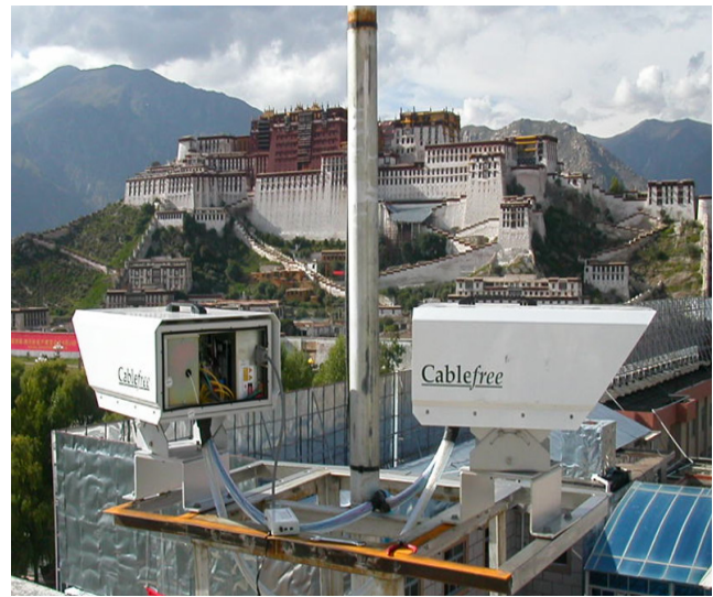
Figure 2: FSO installed in Tibet
