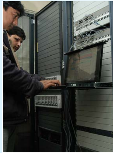
ADSL system equipment
