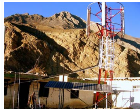
GSM BTS installation at Jomsom
